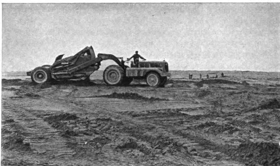
Figure 67. Spreading natural base material—volcanic cinders. (See fig. 74 for view of finished base.)
